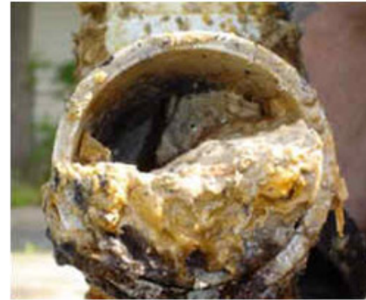
Pipe Clogged with Fat, Oils, & Grease
